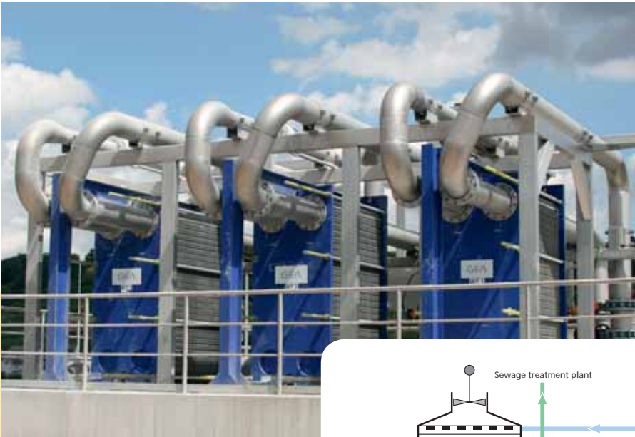
Waste water cooling at Papierfabrik Palm, plant Eltmann
