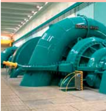
E-on, pumped storage power plant
