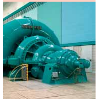
E-on, pumped storage power plant
