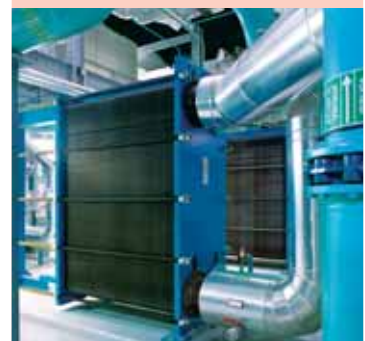
BEWAG, combined heat and power plant Berlin Mitte
