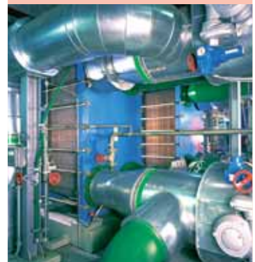
BEWAG, combined heat and power plant Berlin Mitte
